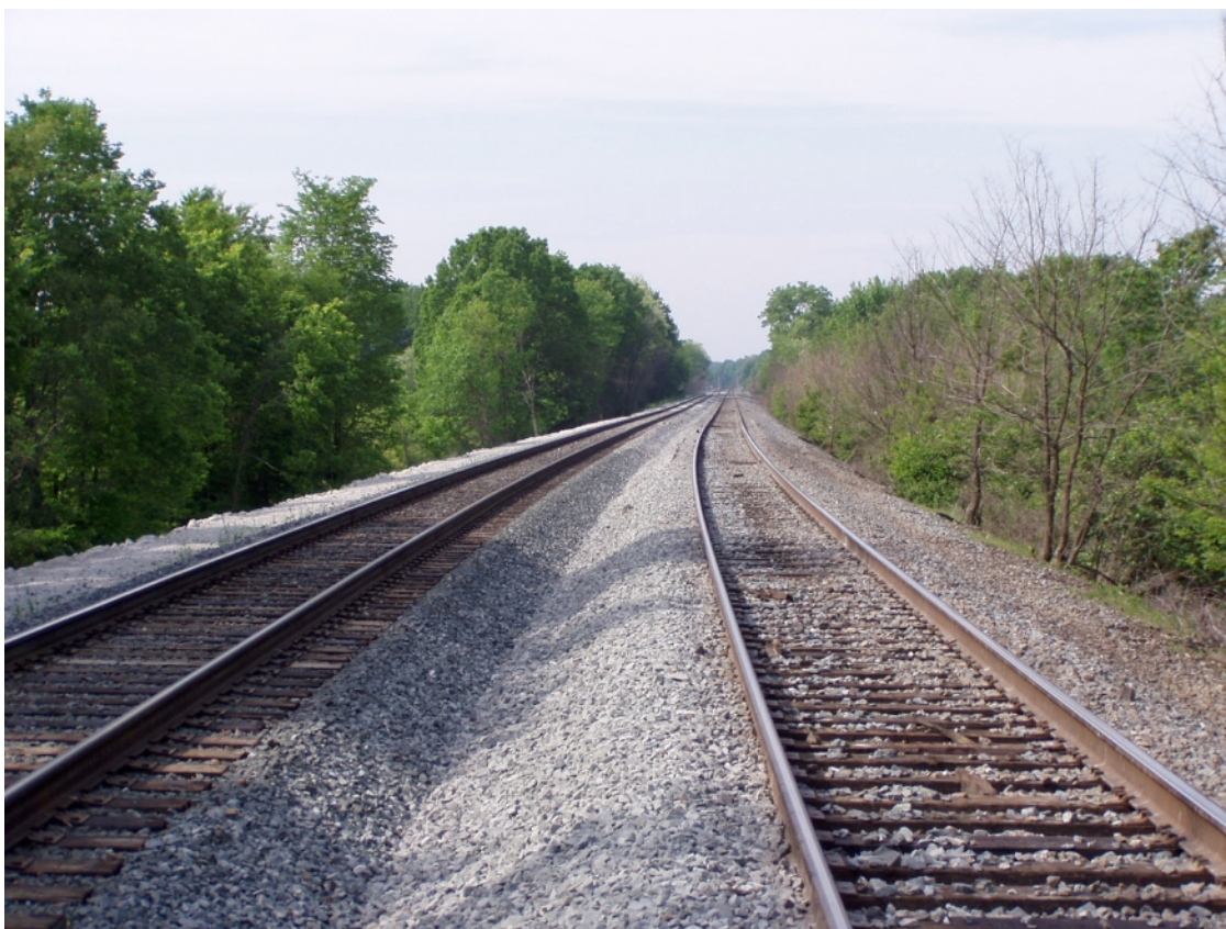
Last year at this time, the double track extension project north of Danville was in full swing. These before and after shots looking southbound at MP 119.5 show the transformation that occurred. Taken in November of 2006 and May of 2008, respectively, they show a new #2 main on the left where there was none before, and a re-invigorated #1 that was formerly just single main track north of the original RA Jct. Now if they would just finish the Winter Ave bridge, this project will be finally DONE. Photos by DN.
