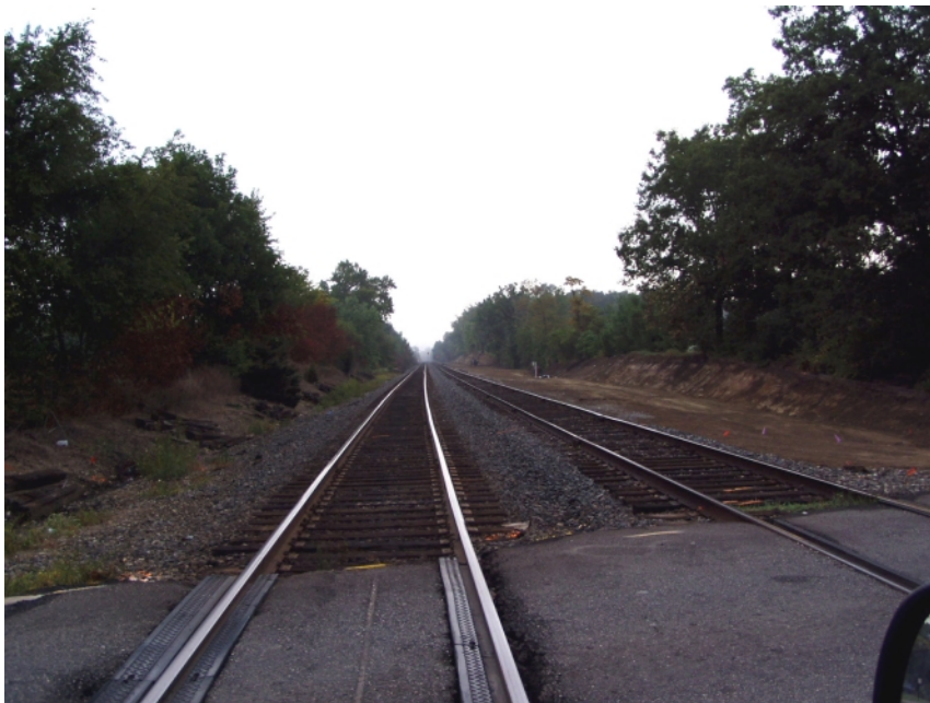
Looking northbound at Liberty Lane, we see the excavated area for the new control point that will govern the universal crossovers planned for this location. The bank was cut back for working room and later a permanent access road.
