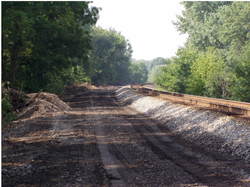
Evidence of heavy equipment working is visible in this south-looking shot just south of MP 119, which is about the mid-point of the siding extension project. Note the piles of "mulch" rendered by the large chipper/shredder that dealt with all the tree and brush debris. They have since added more soil to the east side of the fill in this area.
