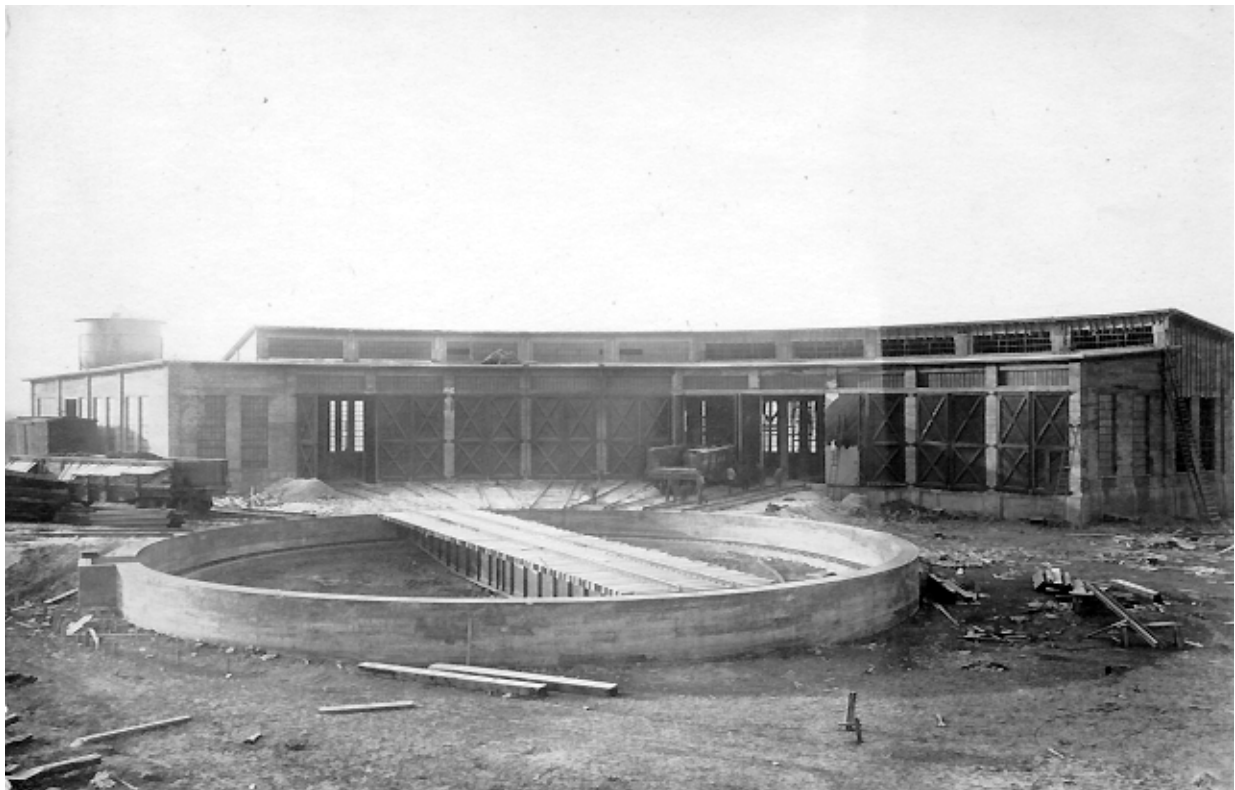
Below: Outside view of the nearly completed roundhouse with 80 foot turntable in place. Some fill is present around the pit ring. Tracks are laid in for stalls 1-7. New water tower has been installed, but no well drilled yet.
