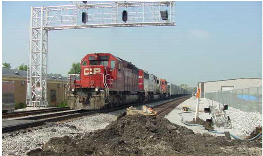
Eastbound CP Rail train at Chatham Street on future No. 2 track. New No. 1 under construction west of Chatham. Area to right was purchase of right of way for new drainage system. Note building in background, right of way offsets around building.
